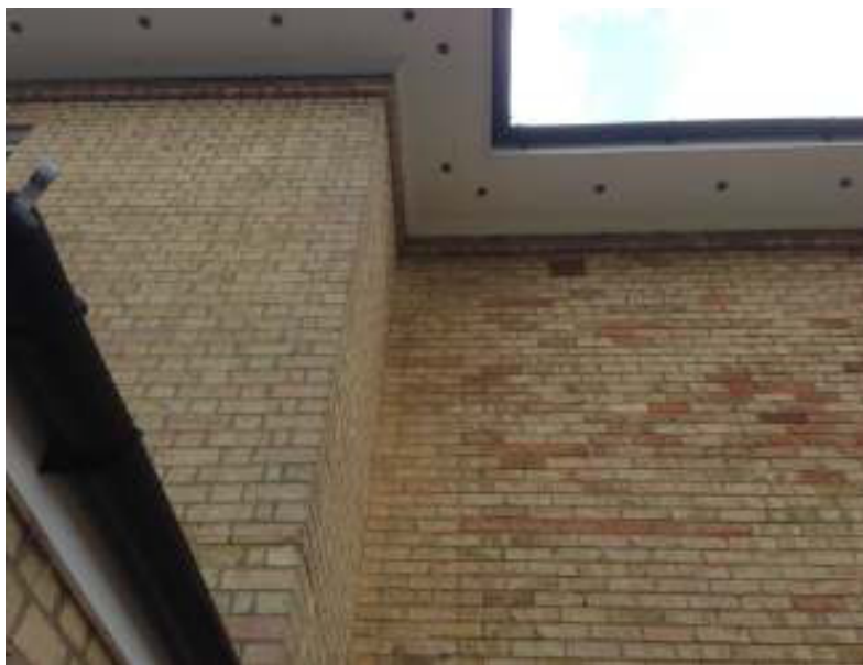
Original Villa with simple over-sailing courses copied on the modern stretcher bond, cavity wall extension using reclaimed bricks and four-board copy of the original soffit
