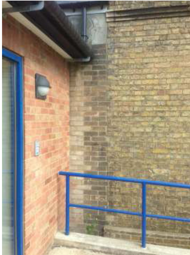
Detail of the toothed-in brickwork to west of original house showing three phases of change during the 1950s and 1960s to the original Victorian building
